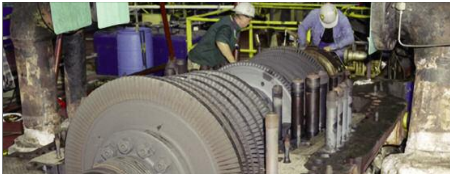
Power plant turbine unit. Courtesy: TVA and EPRI.
