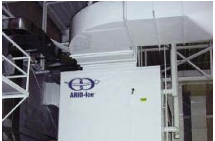
Indoor installation rated at 12,000 SCFM.
