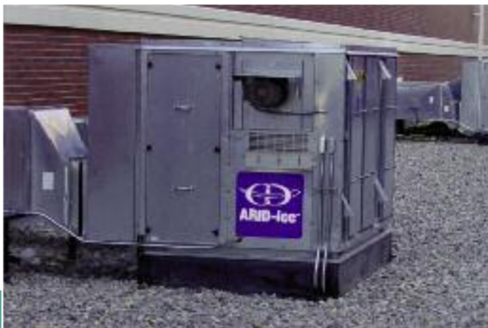
Rooftop installation rated at 5,500 SCFM
