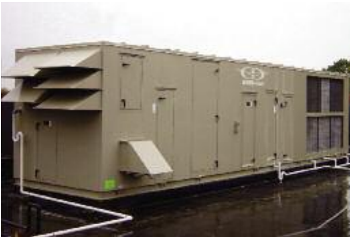
Rooftop installation rated at 10,000 SCFM
