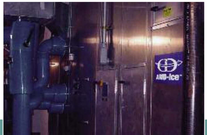
Indoor installation rated at 45,000 SCFM.
